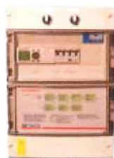
Veto regeling-controle panelen
